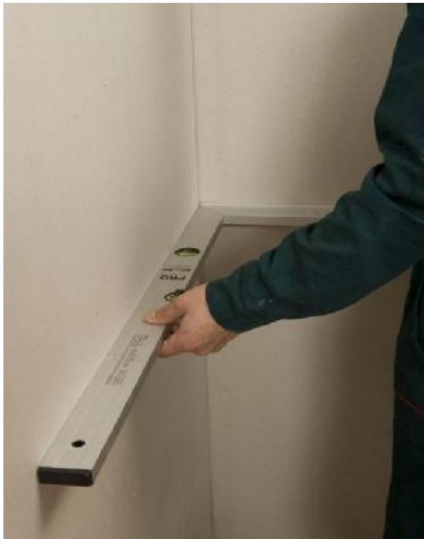
Fig 5. Checking deviation of intersecting planes from the angle specified in the documentation.
