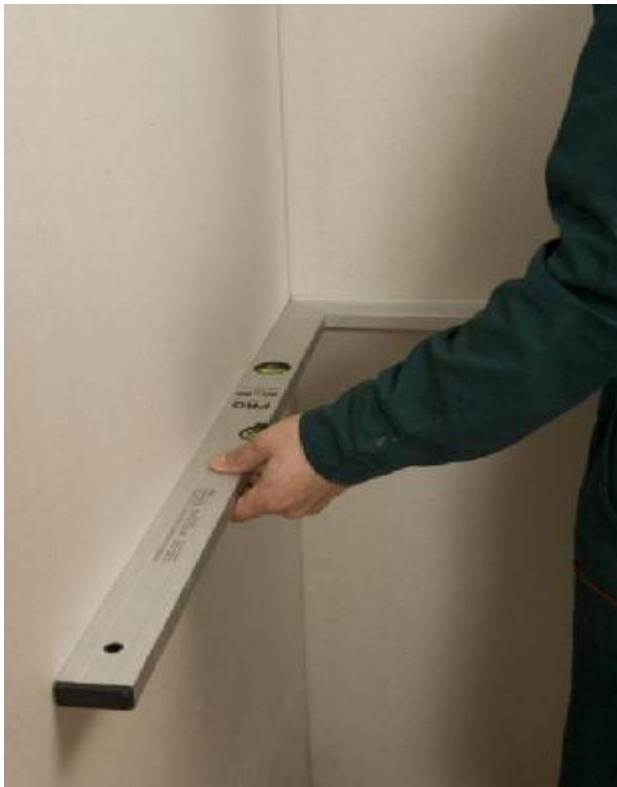
Fig 12. Checking deviation of intersecting planes from the angle specified in the documentation.
